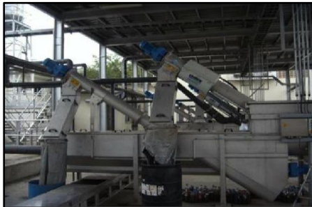
Septage Acceptance Unit
